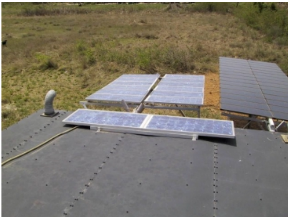
Figure 6.6. The PV-panel of the two wood dryer. The PV arrays are movable in order to allow for cleaning of the PV-panels and later tracking of the sun.
