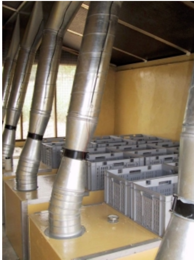
Figure 6.2. The five drying units inside the building containing the solar crop dryer.
